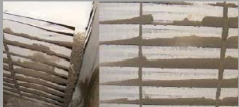
Heating, Ventilation and Cooling (HVAC) condenser after ~32 mm of wet ash was applied over ~ 4.5 hours
