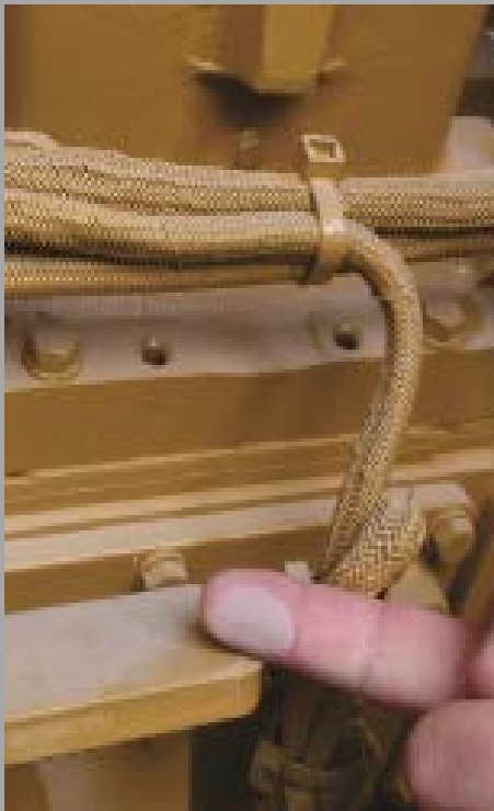
Ash deposited on the engine block of a generator within the new 20MW generator farm. Deposited ash can potentially be ingested by the engine air filter which may lead to stalling.
