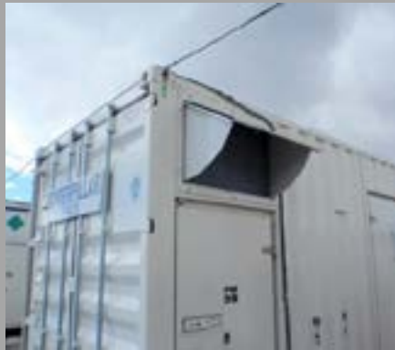
Hood to protect air intake from ashfall for GenSet equipment in Bariloche, Argentina, following 2011-2012 eruption of Cordón Caulle volcano, Chile.
